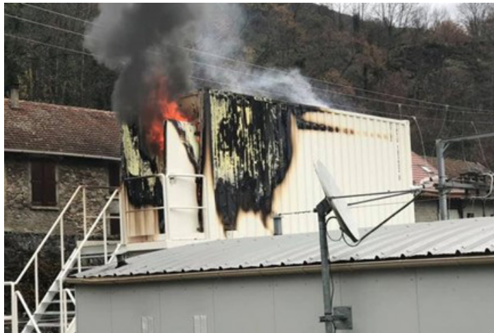
Figure 25. A BESS container lithium-ion fire at an electric substation in Ariège, France
