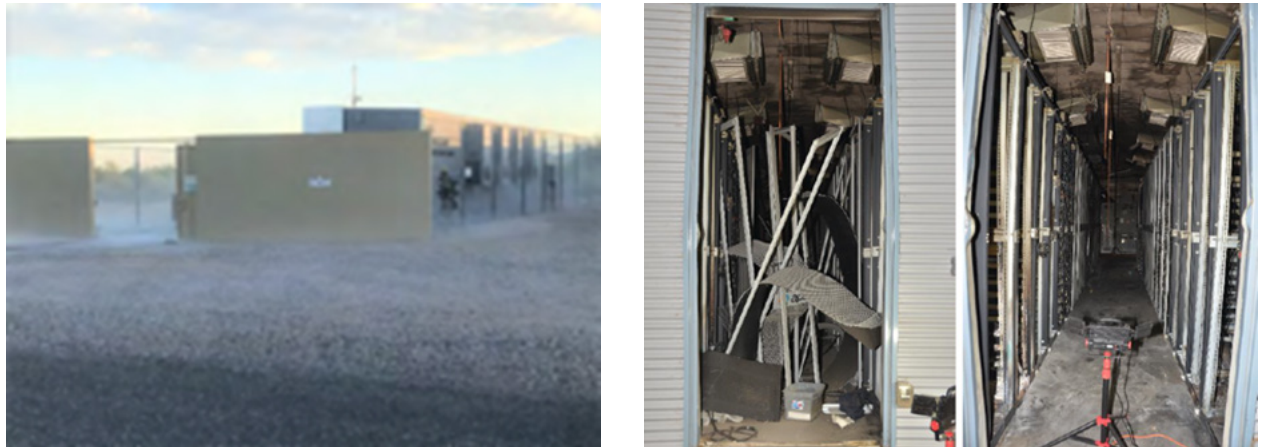
Figure 18. Photo (left) of the APS BESS and low-lying vapor cloud upon the arrival of the Emergency Responders; photo (right) damage to modules and racks inside the BESS container (UL Report Photos)
