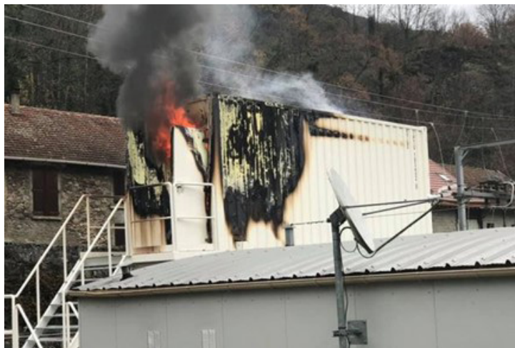
Figure 25. A BESS container lithium-ion fire at an electric substation in Ariège, France
